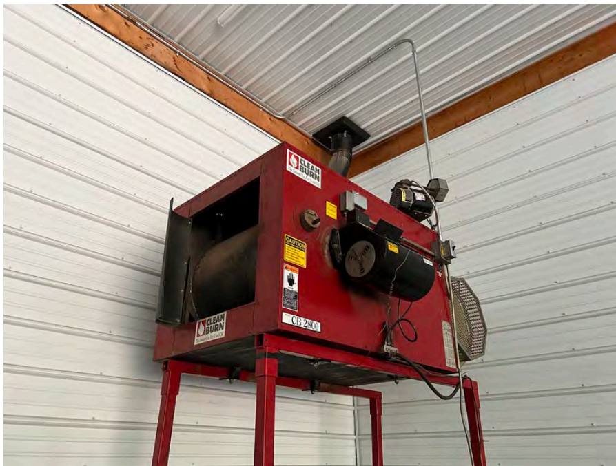
Photo 42 : Waste oil heating system in Building Four
