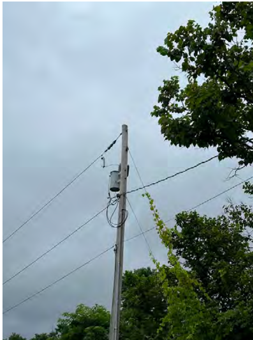
Photo 66 : Pole-mounted transformer on Subject Property
