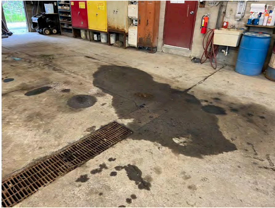
Photo 17 : Representative staining in Building One
