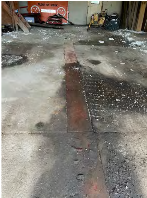
Photo 32 : Capped trench drain in Building Three
