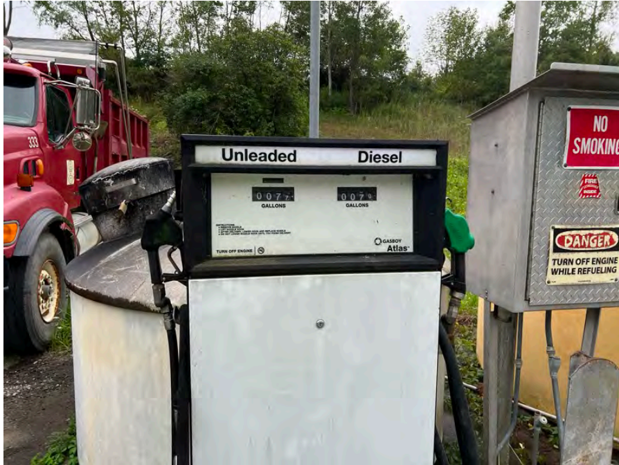
Photo 48 : Gasoline and diesel dispensers
