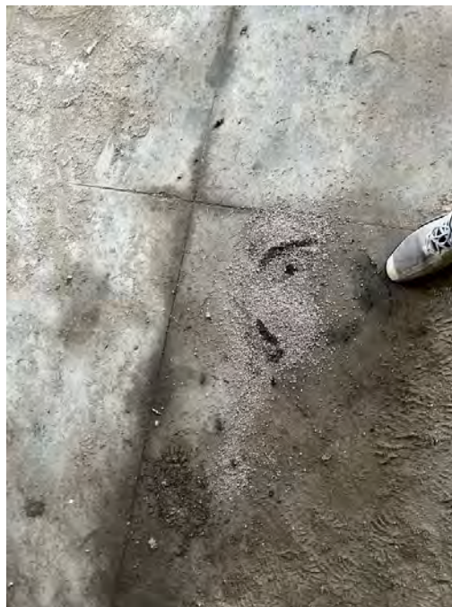
Photo 38 : Representative staining in Building Four
