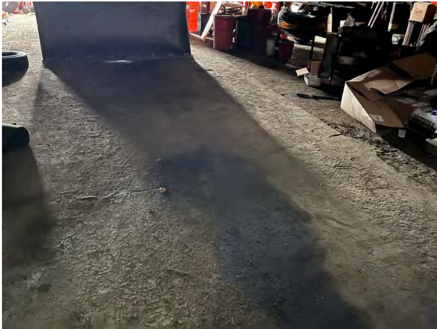
Photo 22 : Representative staining in Building Two
