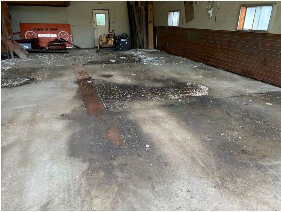
Photo 31 : Representative staining in Building Three
