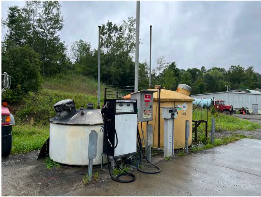
Photo 47 : 3,000-gallon diesel AST and 1,000-gallon gasoline AST on Subject Property
