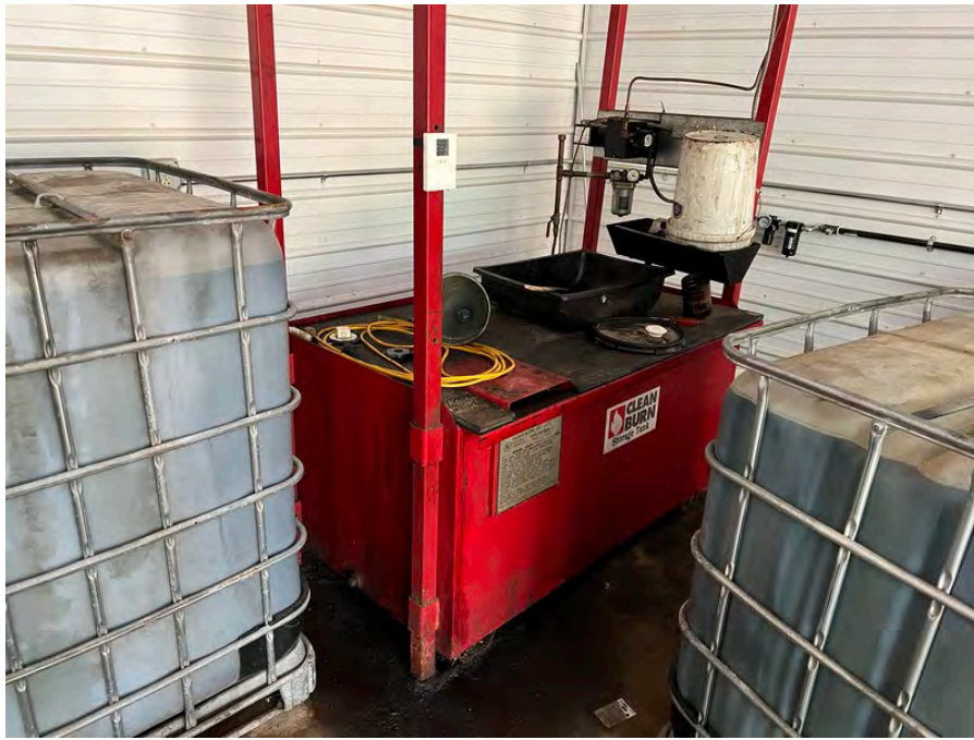
Photo 41 : Waste oil AST in Building
