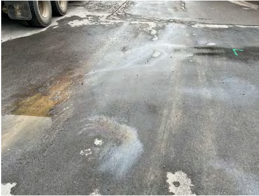
Photo 69 : Petroleum sheen on northern portion of Subject Property
