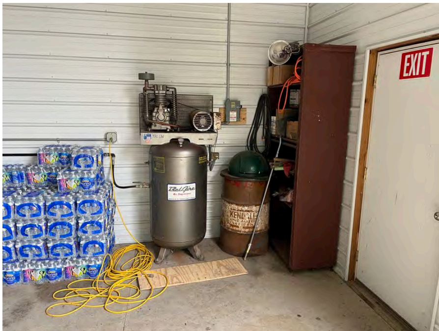
Photo 40 : Compressor in Building Four
