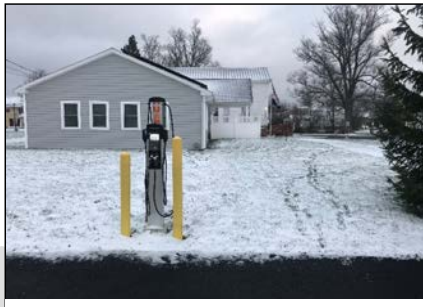
Electric Vehicle Charging Station at the Brooktondale Post Office
