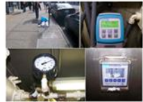
Figure 28. Checkmate from top left - of typical dewatering. 1) flow meter installed, 2) water level meter installed and 3) pressure gauge installed to water line.
