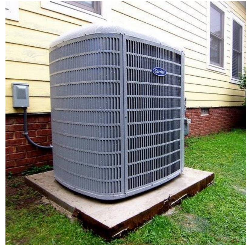
Remote Outside Condenser
