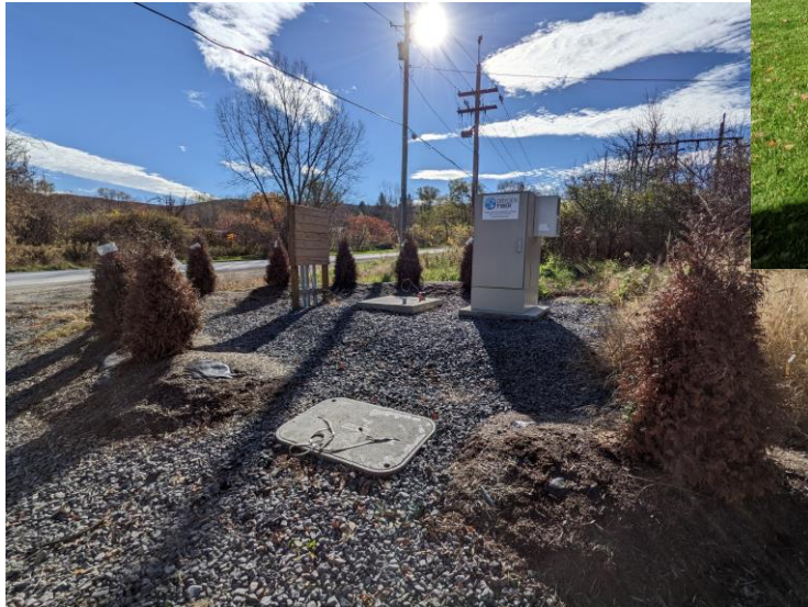
Pinckney Point of Presence (Etna, NY)
